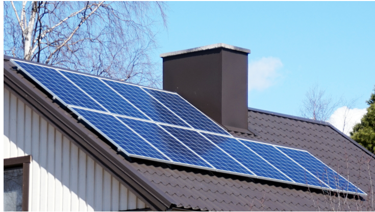
Figure 1.1: Solar panels installed on the roof of a building. Reprinted from energy options, 2019.
