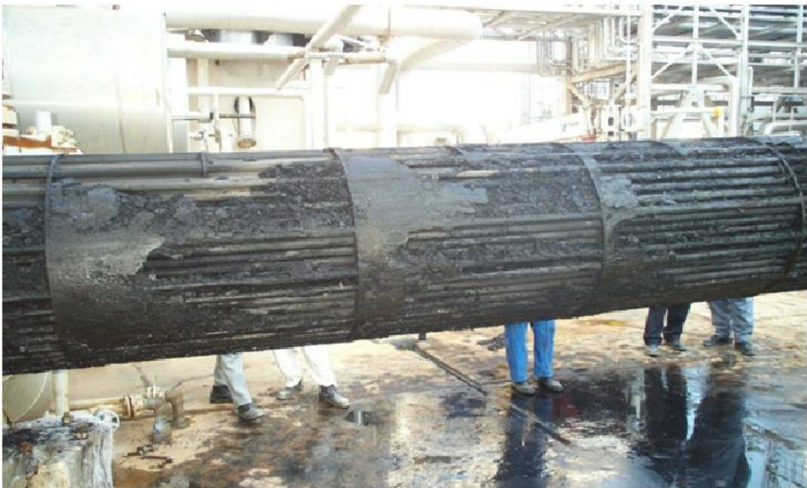
Figure 2. Fouling on the surface of the heat exchanger. (Ibrahim, 2012)
