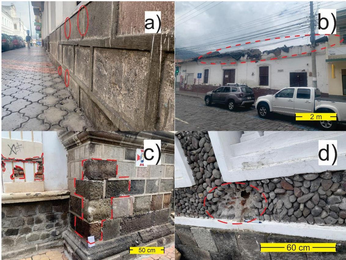
Figure 6. Features induced by material loss in the historical center of Ibarra, a) Mechanical damage, Simon Bolivar & Miguel Oviedo str., b) Erosion, Vicente Rocafuerte & Miguel de Oviedo str., c) Alveolization, Episcopal Chapel, Pedro Moncayo str., d) Missing part, Simon Bolivar & Eusebio Borrero str.
