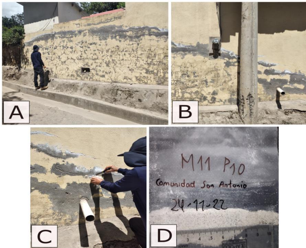
Figure 16. House wall with crystals in the San Antonio community (See location in Figure 1) (A). A deteriorated light pole with exposed iron bars (B). Obtaining a mineral sample from the wall near the drainage (C). Sample M11P10 obtained (D).
