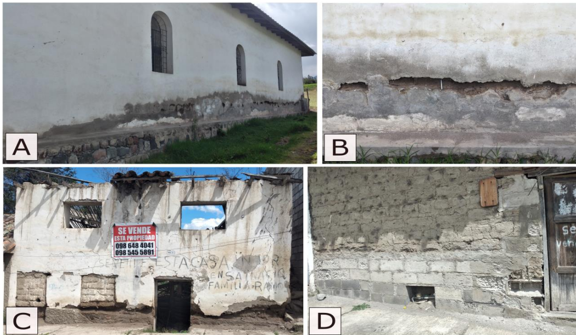
Figure 17. Church wall with exterior degradation (A). The degree of degradation of the wall (B). Old house with significant degradation (C). The combination of construction materials and their degradation (D).
