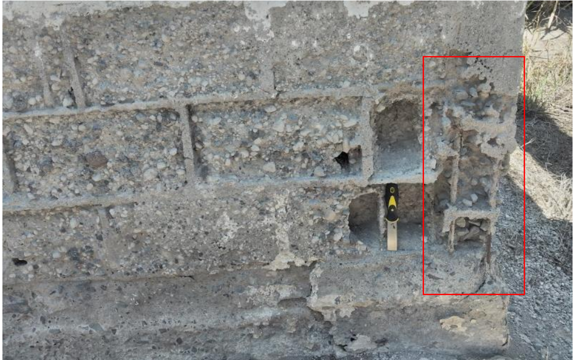
Figure 3. The building's infrastructure appears to have a significant amount of corrosion. The concrete blocks are already breaking apart, and the iron bars are exposed, increasing the likelihood of a potential collapse in the future. The photo was captured in an abandoned building located in Tapiapamba (See location in Figure 1).
