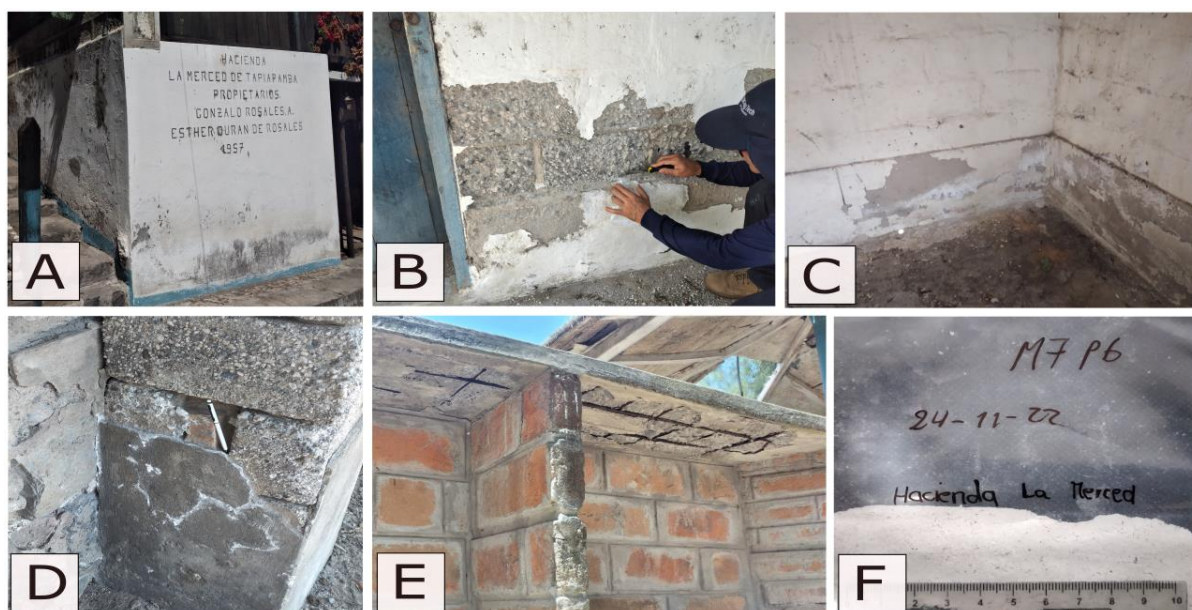
Figure 13. La Merced Farm construction from 1957 (See location in Figure 1) (A). The sample was taken in a porous material (B). White crystals were identified in the wall of an abandoned house (C). Concrete block pillars with salt crystals (D). Iron is revealed beneath a concrete table (E). Salt sample M7P6
