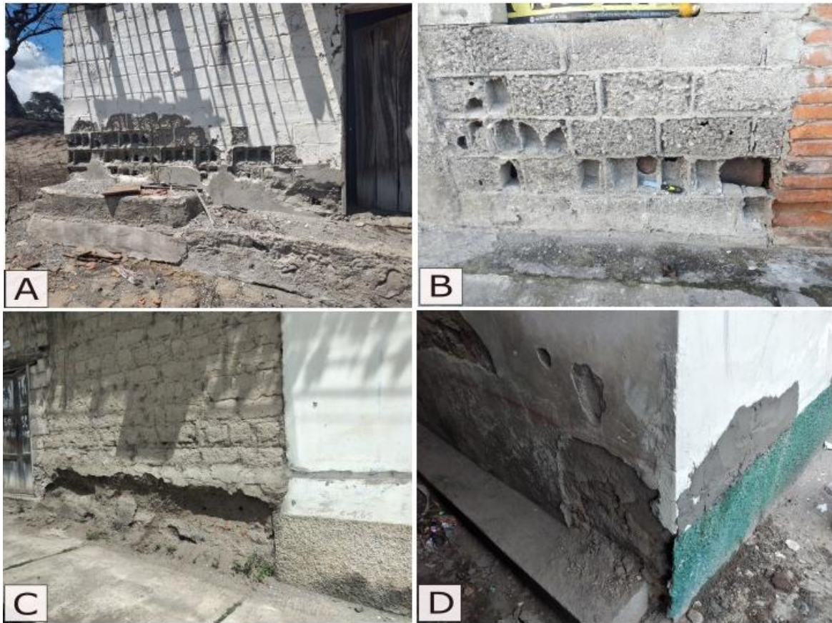
Figure 33. Constructions with deterioration at the base of the walls. Concrete blocks exposed to weathering with high levels of damage (A) (B). There are some missing blocks on a house wall in Urcuquí town, which was damaged by weathering (B)(C). The wall underwent recent repairs, with cement patches applied to cover holes that resulted from deterioration (D).
