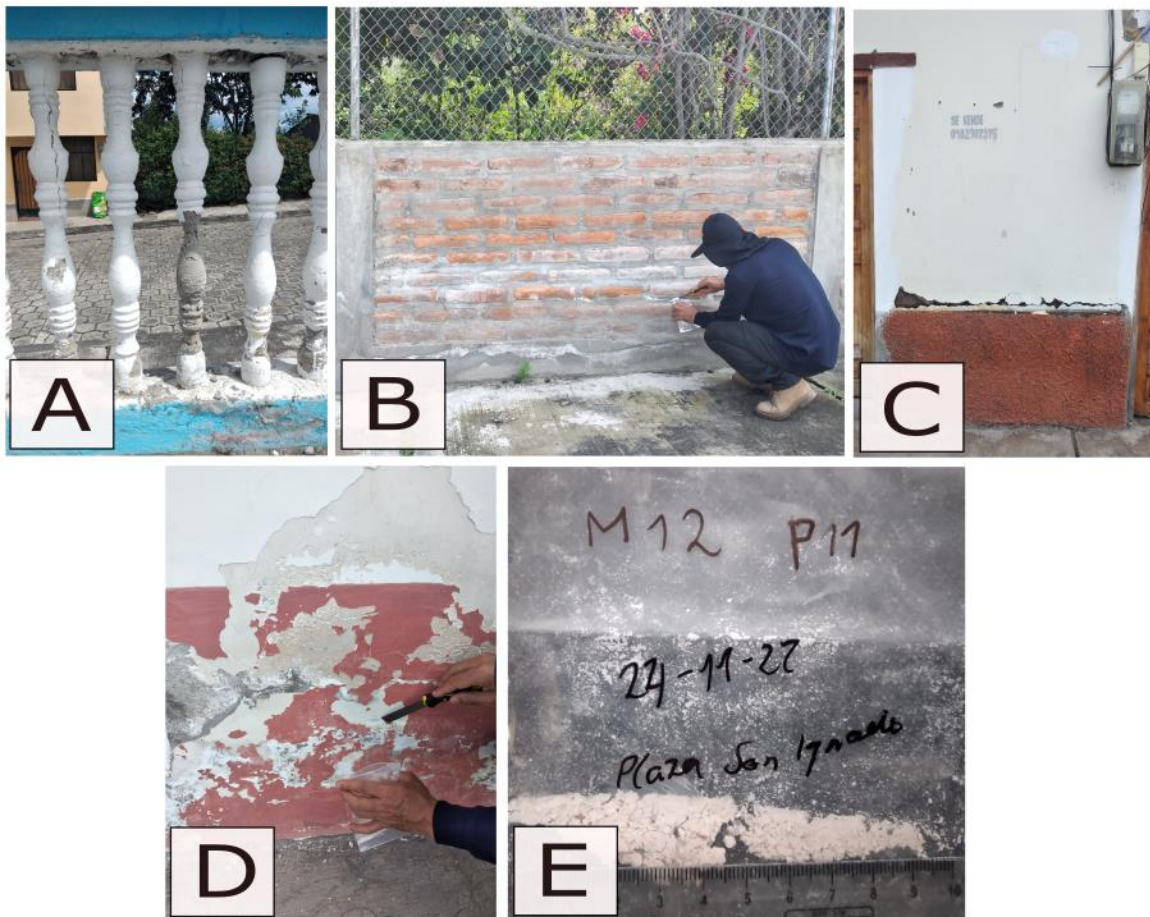
Figure 18. Deteriorated handrails in the San Ignacio Plaza (See location in Figure 1) (A). The sample was taken from a brick wall (B). Base wall with deterioration-caused fractures (C)(D). The sample was taken M12P11
