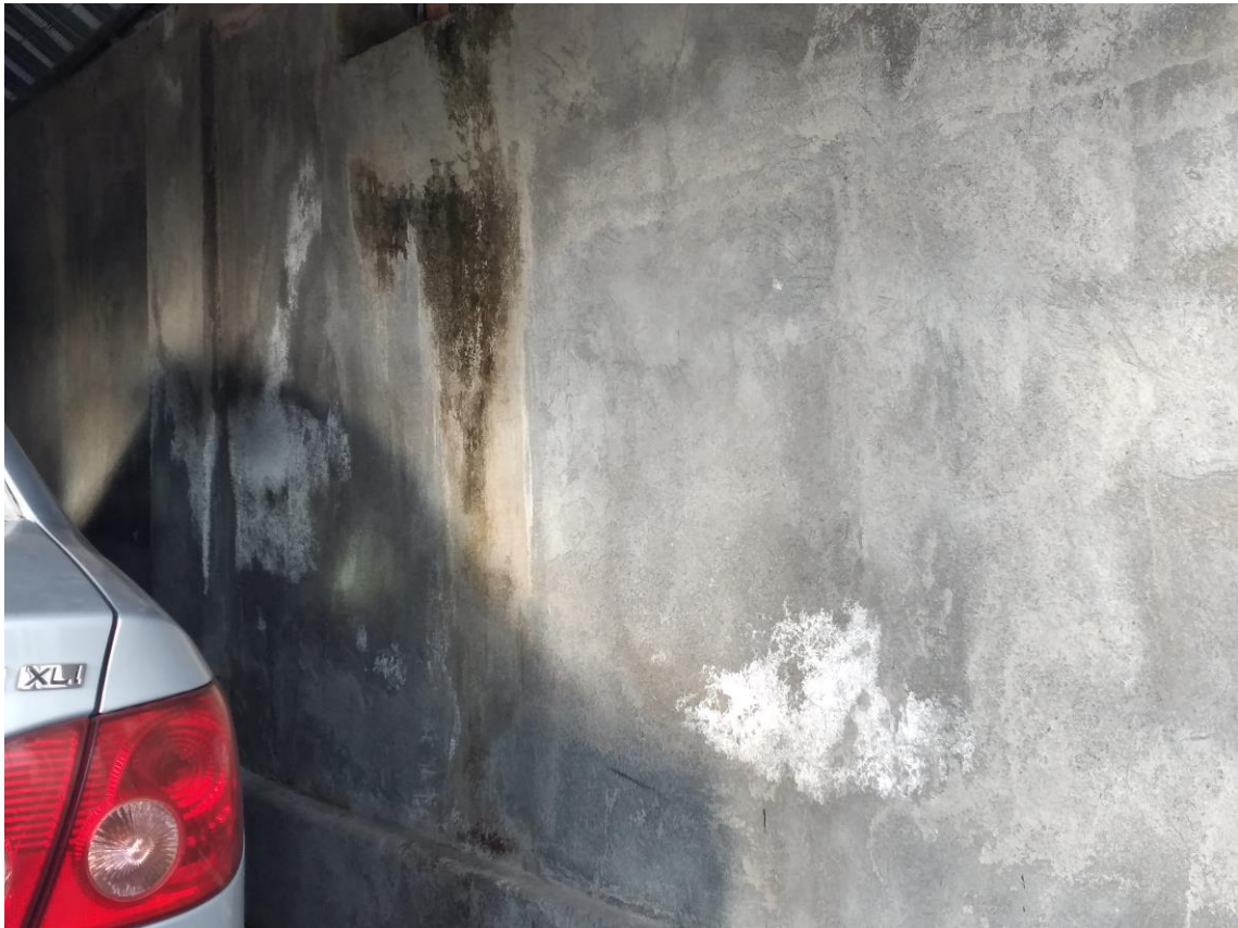
Image 9. The white and black spots on the wall indicate the presence of water filtration, wetness, and CO2.
