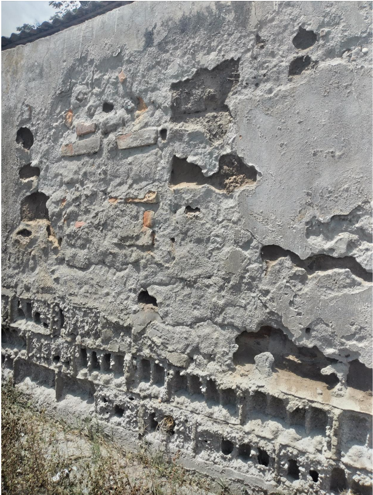
Image 7. The wall has significant deterioration at the base and a moderate level higher up. It has been patched with brick and concrete to cover large holes. The blocks have shrunk by half due to their significant deterioration.
