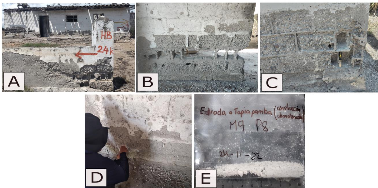
Figure 14. Abandoned construction in Tapiapamba (See location in Figure 1) (A). Concrete block deteriorated (B). Iron exposed in concrete block construction (C). Sample-taking process (D). Salt sample M9P8(E).
