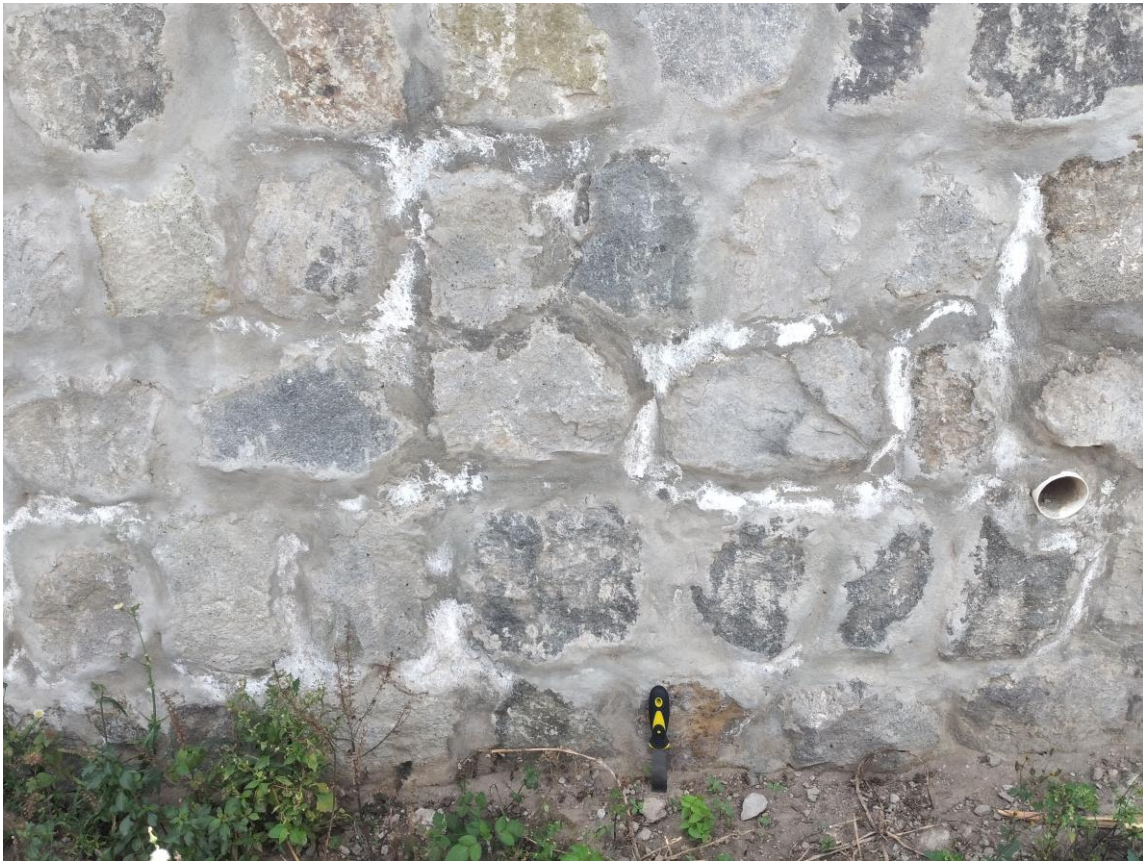
Image 4. Rock blocks are surrounded by white crystals growing in the mortar.
