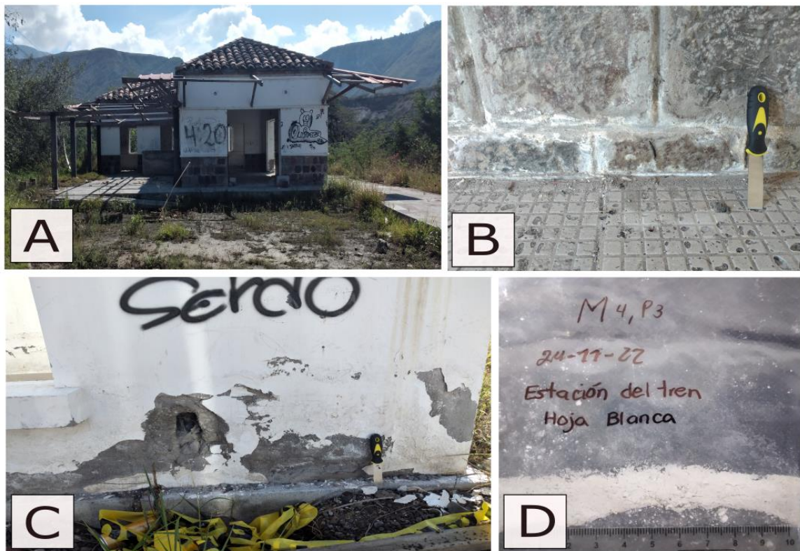
Figure 10. Hoja Blanca Train Station (See location in Figure 1) (A). The internal wall presents salt crystallization (B). Abandoned and deteriorate building (C). M4P3 Sample taken from the inner wall (D).
