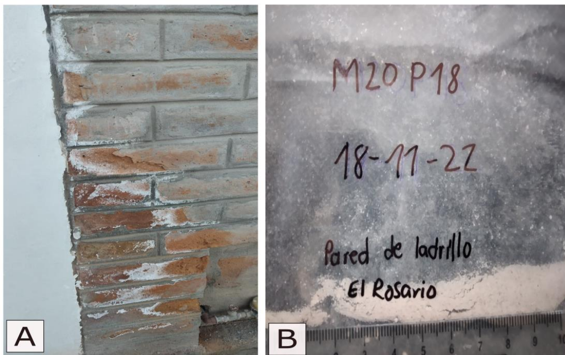
Figure 26. Brick wall with degradation and white minerals growing in El Rosario neighborhood (See location on Figure 1) (A). Sample taken from the wall analyzed (B).
