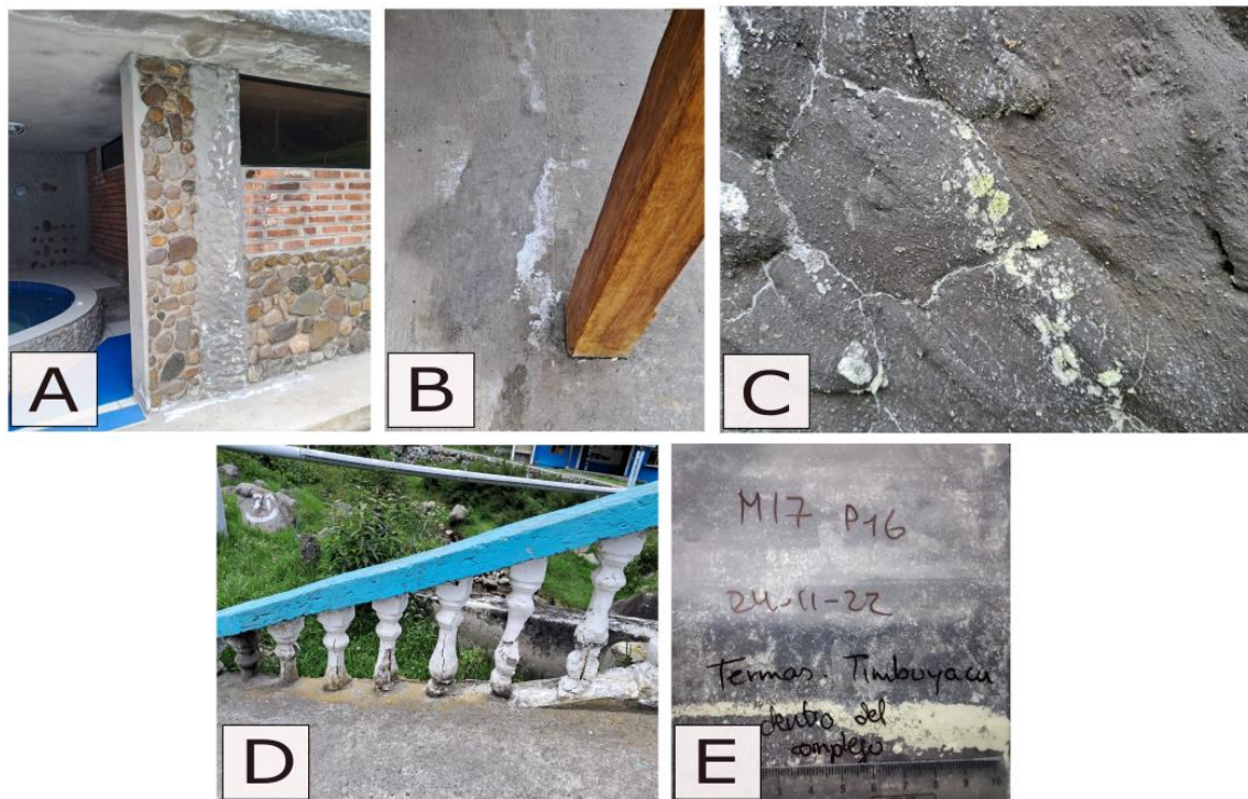
Figure 23. Timbuyacu Resort walls with salt crystals (See location in Figure 1) (A), Salts are growing in the soil (B), Cement railing pillars deteriorated (C), and Sample (M17P16) was taken from this resort.
