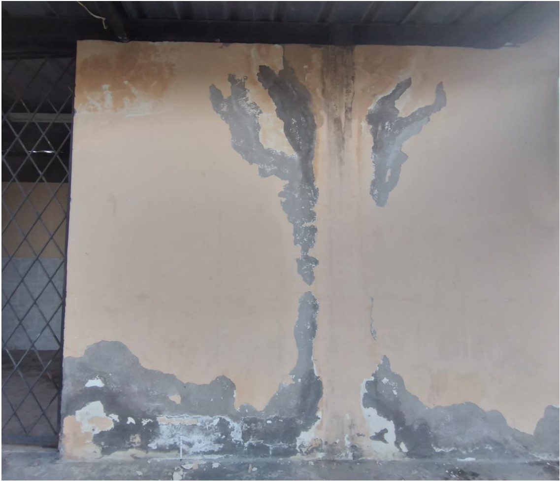
Image 8. Filtration of water could lead to the degradation of paint, forming salt crystals at the bottom of the wall.
