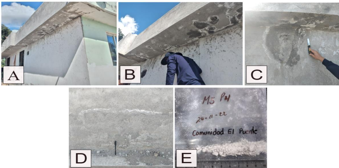
Figure 11. House in El Puente Community with possibly salt crystals (See location on Figure 1) (A). Identifying the existence of crystals in construction (B). Taking the mineral sample from the wall (C). Crystals at the base of the wall(D). Sample M5P4 taken (E).
