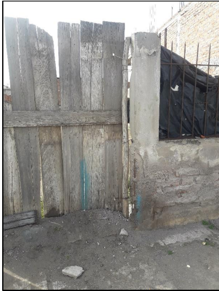
Figure 14. Several Cases of Salt Growing. The figure shows a several cases of slat growing where the mortar that cover the walls and the concrete that covers the iron rods have been removed. Likewise, the iron rods exposed in the lower part of the column show signs of oxidation. Even though the iron rods are exposed, no flexion of the concrete column is seen (Author).
